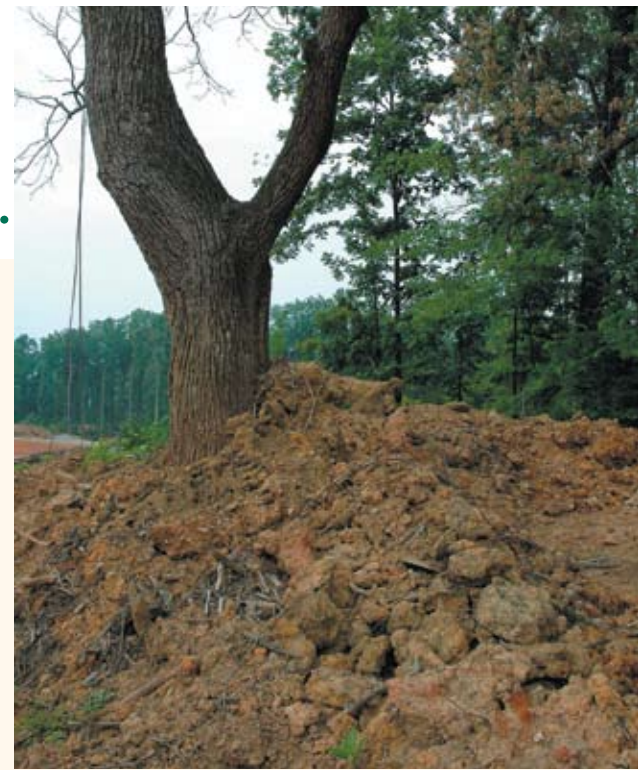
This dozer filling is an example of detrimental grading.
